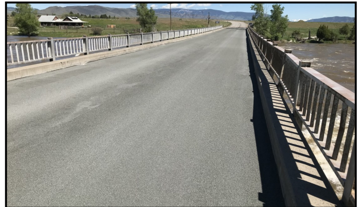
Top: Final Grade in Gravel Section Bottom: Completed Epoxy Overlay on Yellowstone Bridge
