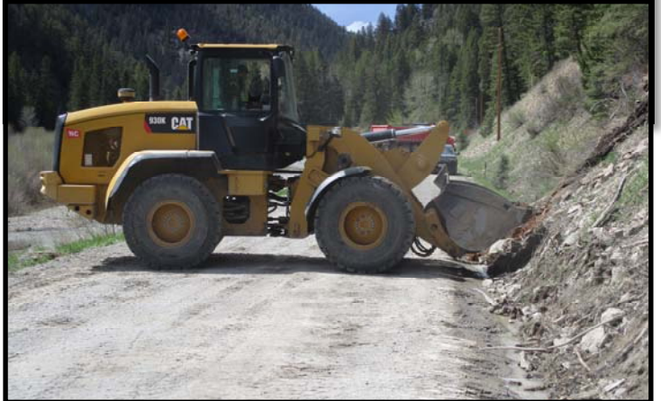
Above: Subexcavation and ditch reconditioning work in the gravel section of the project.
