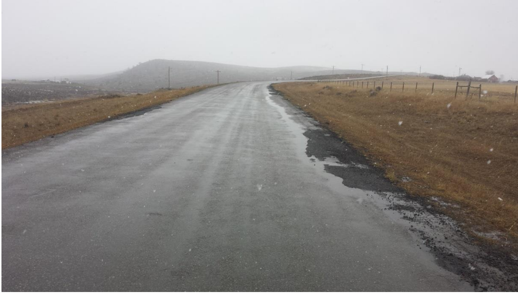
1. Shields River Road: Typical shoulder failure
