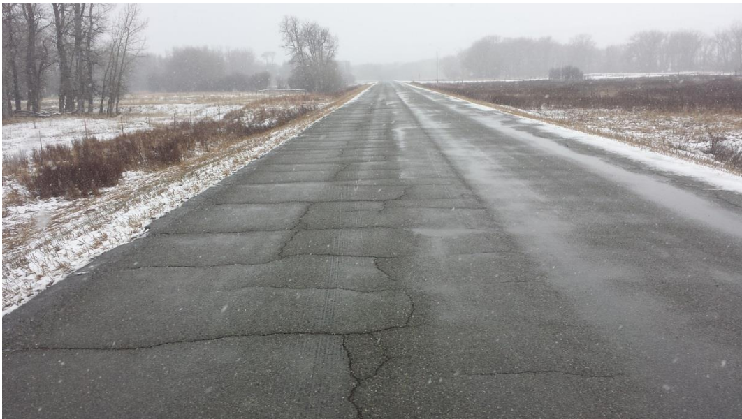
4. Typical traverse cracks at 5'-15' intervals with intermittent longitudinal cracking
