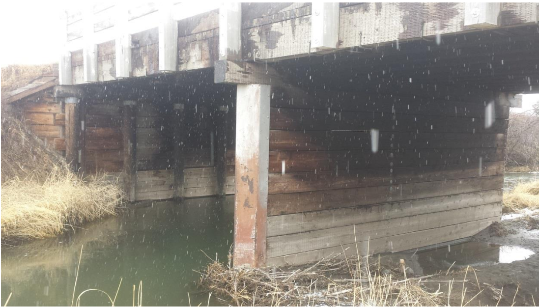
6. Typical structure condition: driving surface in poor condition but structurally sound and may require some safety improvements such as impact barriers, etc.
