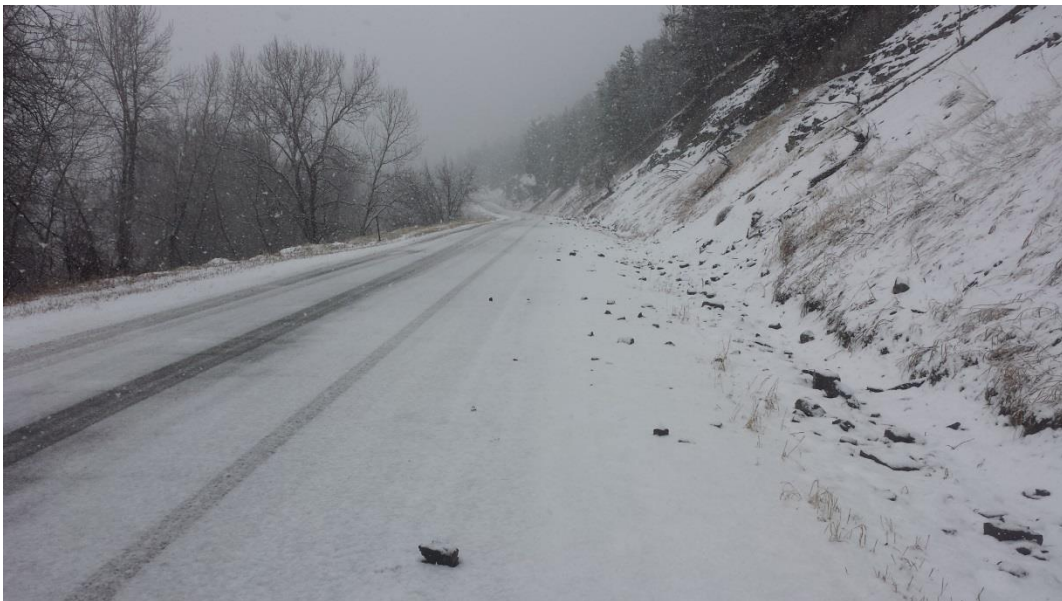
2. Roadside rock fall at area of hill subsidence
