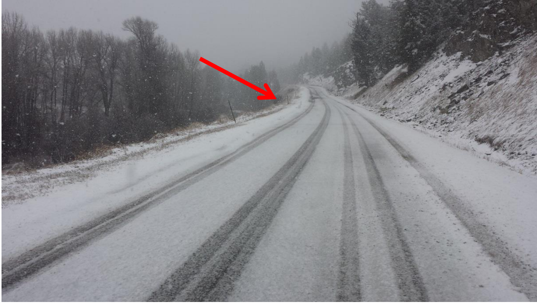
3. Roadway adjacent to River and Hill subsidence requiring roadway reconstruction with stabilization
