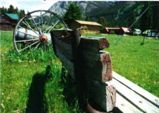
Silver Gate - failing benches - remove immediately
