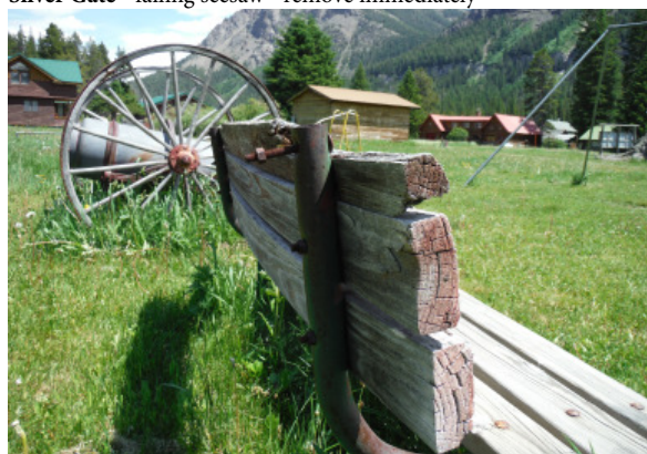
Silver Gate - failing benches - remove immediately
