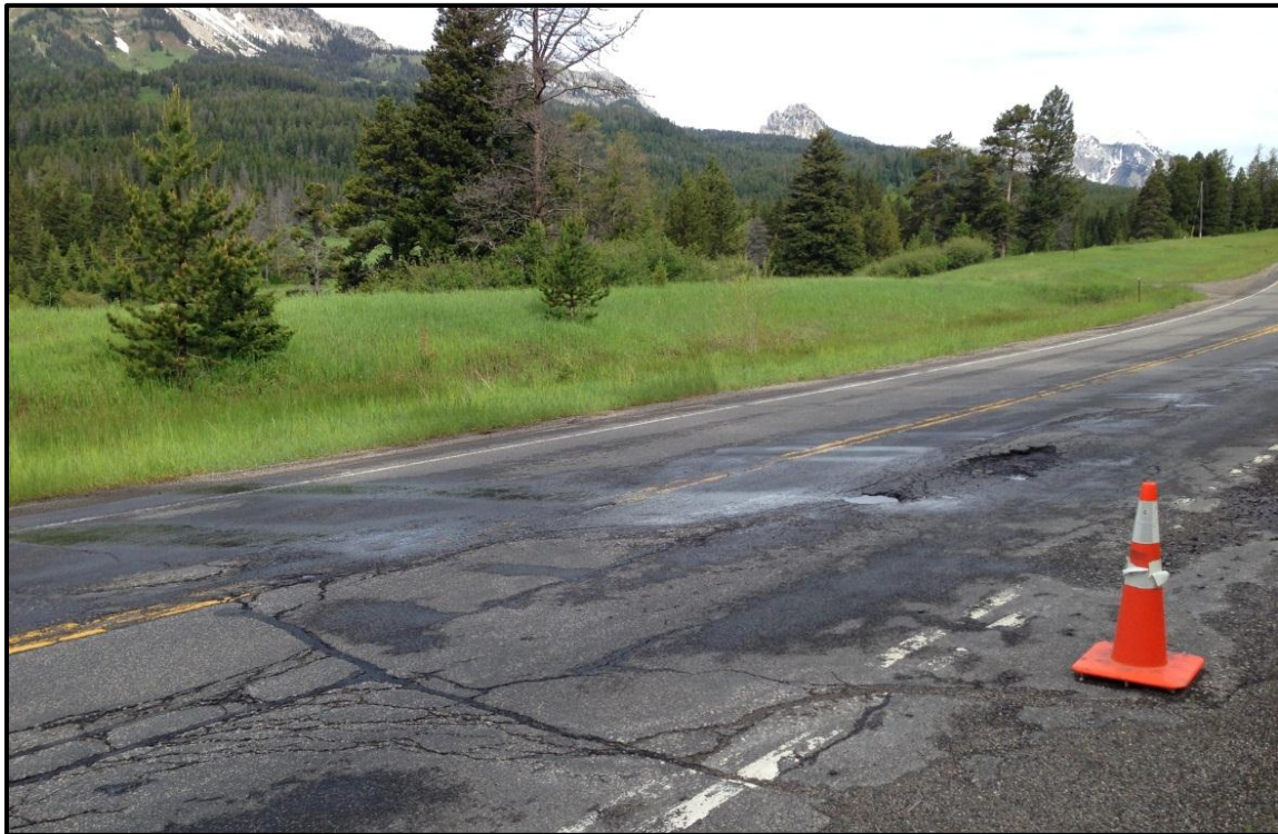
Photo 64. Looking at pavement deterioration due to saturated subgrade on MT 86. RP 15.7.
