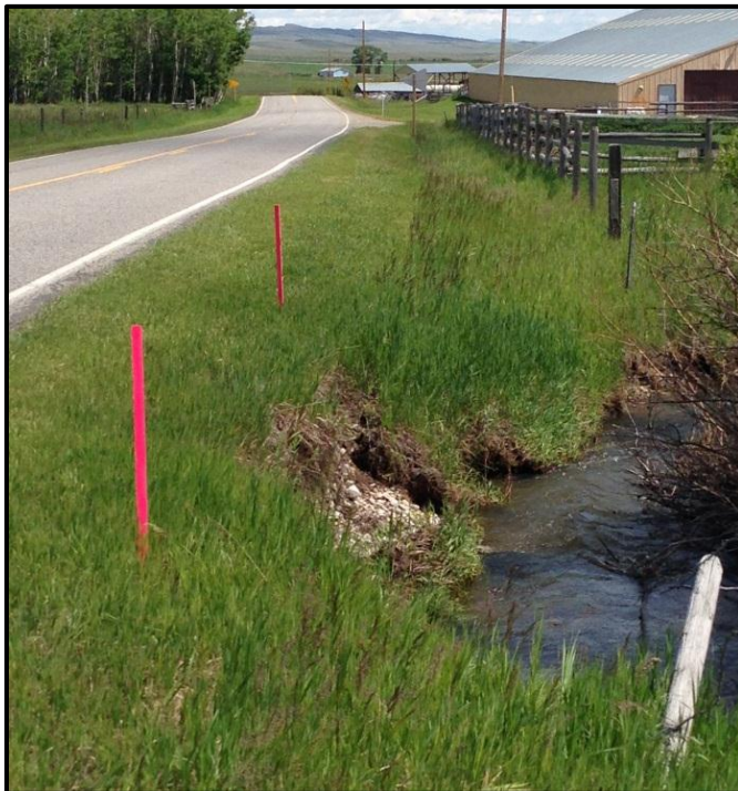
Photo 82. Looking at eroded bank of Carrol Creek. RP 26.8.
