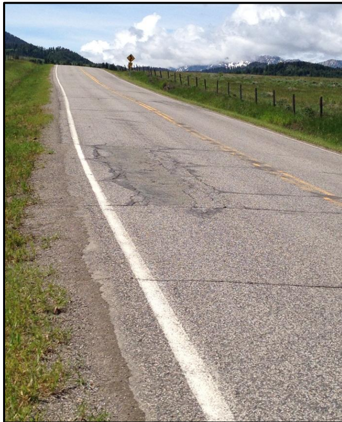
Photo 78. Looking at insufficient sight distance due to horizontal and vertical curves on MT 86. RP 24.7.
