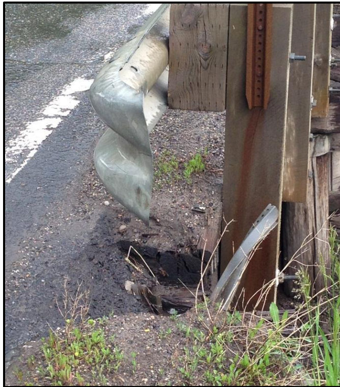
Photo 54. Looking at eroded abutment on a MT 86 bridge crossing an unnamed tributary to Bridger Creek. RP 7.9.
