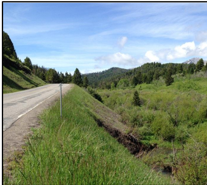
Photo 74. Looking at unprotected substandard fill slopes and substandard back slopes on MT 86 due to embankment erosion on Cache Creek. RP 22.7.
