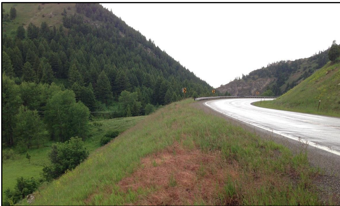
Photo 50. Looking west on MT 86 at insufficient sight distance due to horizontal curves. Unprotected substandard fill slopes and substandard back slopes are also visible. RP 4.8.
