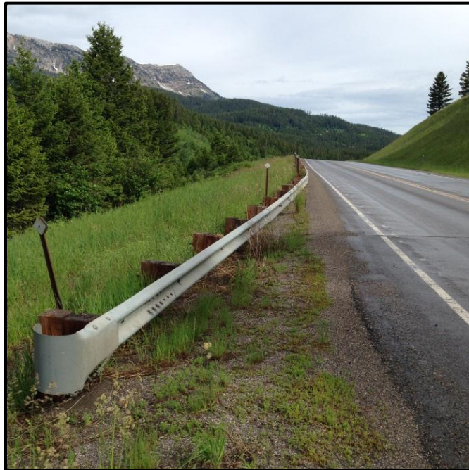
Photo 62. Looking north at substandard guardrail (insufficient height and end treatment) and substandard back slopes on MT 86. RP 13.8.
