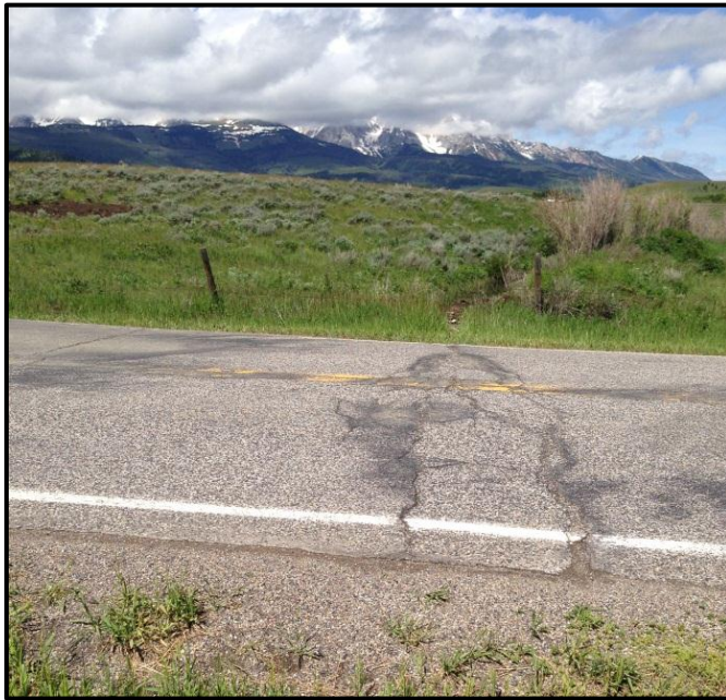
Photo 77. Looking at a deteriorated roadway due to a plugged culvert on an unnamed tributary to Cache Creek. RP 24.7.
