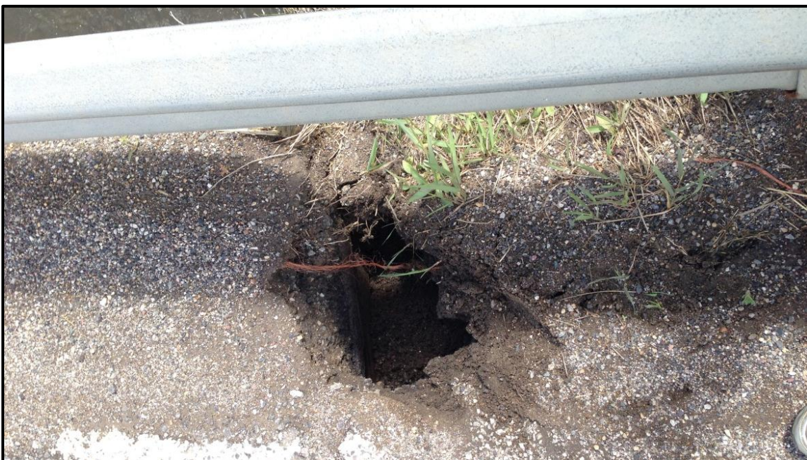
Photo 86. Looking at erosion at Carrol Creek bridge abutment. RP 27.1.
