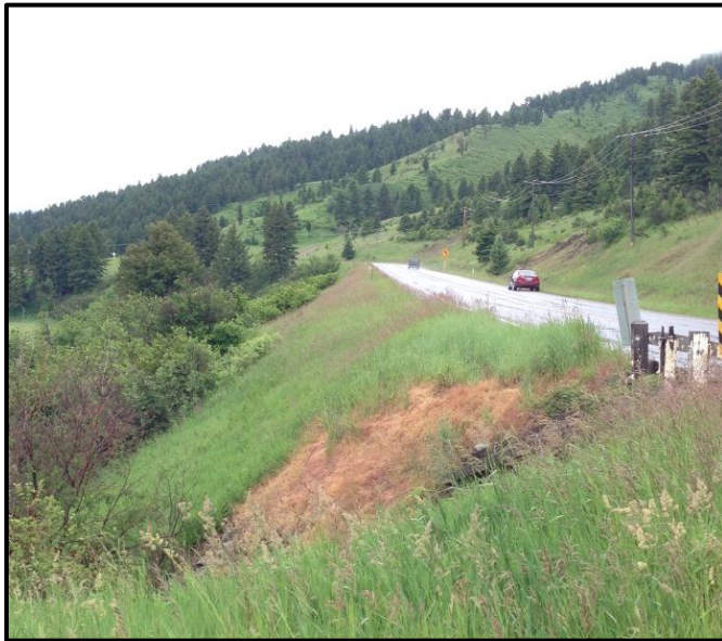
Photo 57. Looking at unprotected substandard fill slopes on MT 86. RP 9.5.
