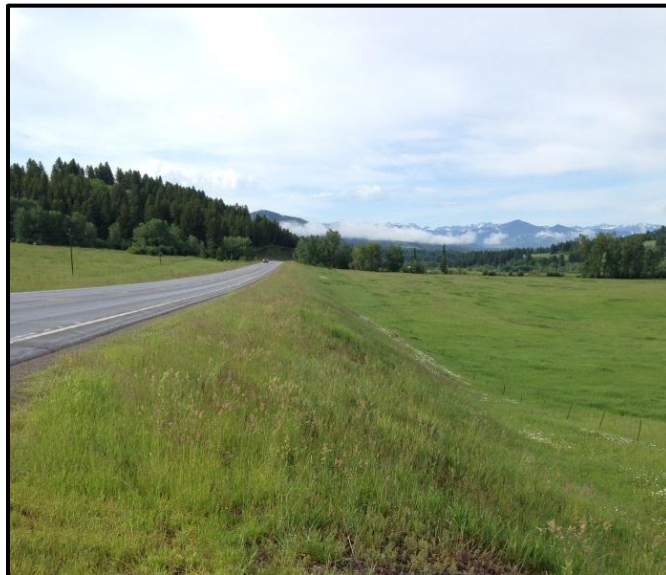
Photo 60. Looking at unprotected substandard fill slopes on MT 86. RP 12.6.
