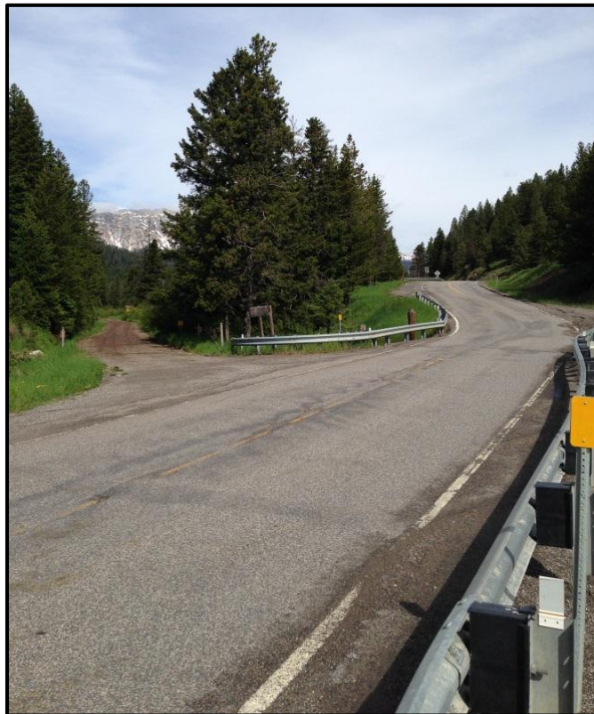
Photo 68. Looking at insufficient sight distance due to horizontal and vertical curves on MT 86 near Brackett Creek. RP 18.8.
