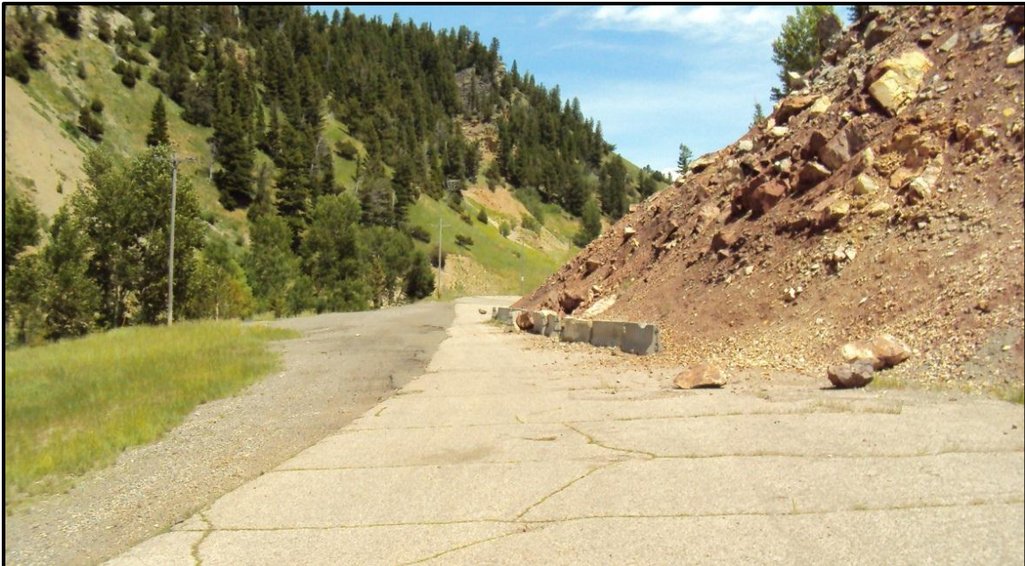
Photo 6. Looking east at a rock slide associated with abandoned quarry, south of MT 86. RP 4.4.
