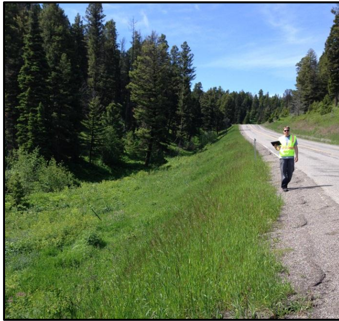
Photo 73. Looking at unprotected substandard fill slopes and substandard back slopes along MT 86. RP 21.0.
