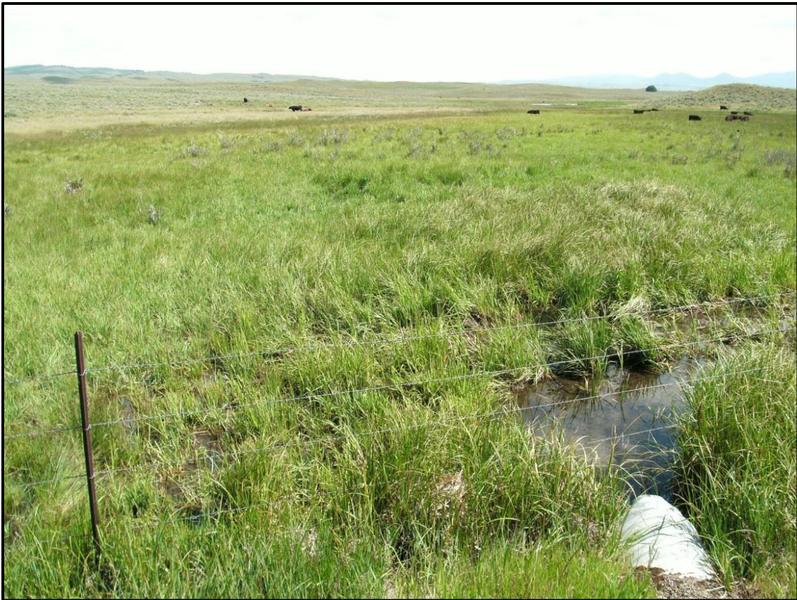
Photo 32. Looking north on an emergent wetland and culvert, north of MT 86. RP 31.0.
