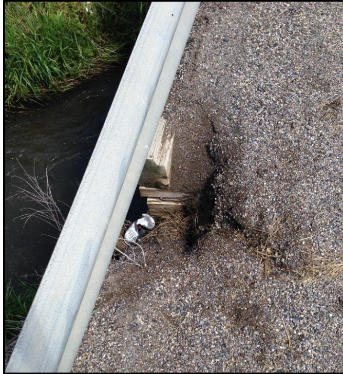
Photo 87. Looking at erosion at Carrol Creek bridge abutment. RP 27.1.
