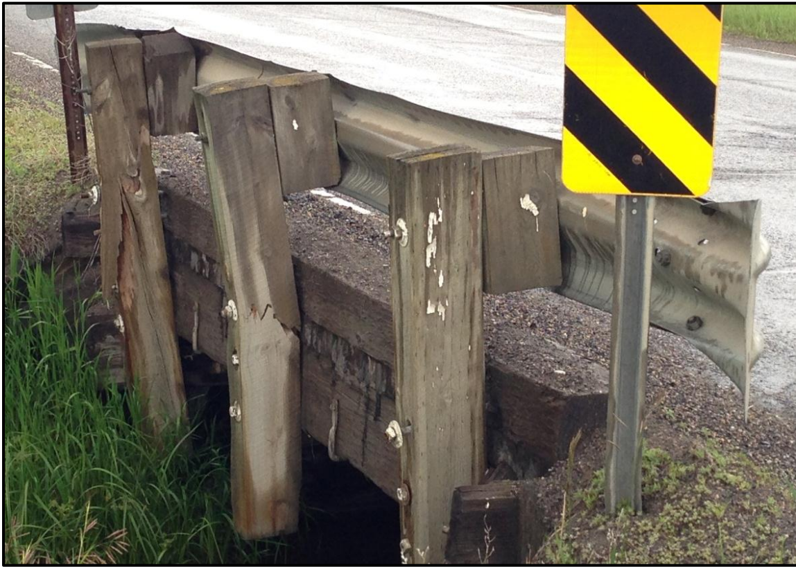
Photo 51. Looking at damaged guardrail on MT 86 bridge crossing Place Creek. RP 6.8.
