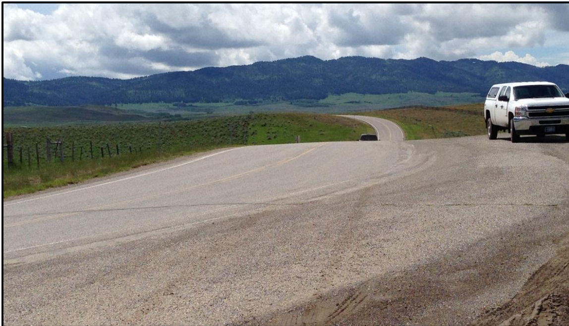
Photo 92. Looking at insufficient sight distance due to horizontal and vertical curves on MT 86. RP 28.9.
