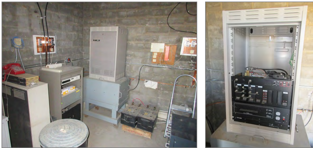
FIGURE 12 North Hill Radio Equipment
