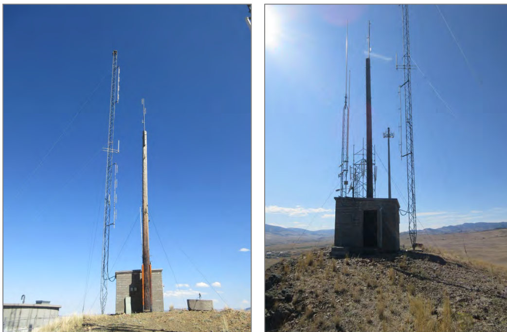
FIGURE 11 North Hill Towers, Pole, and Shelter
