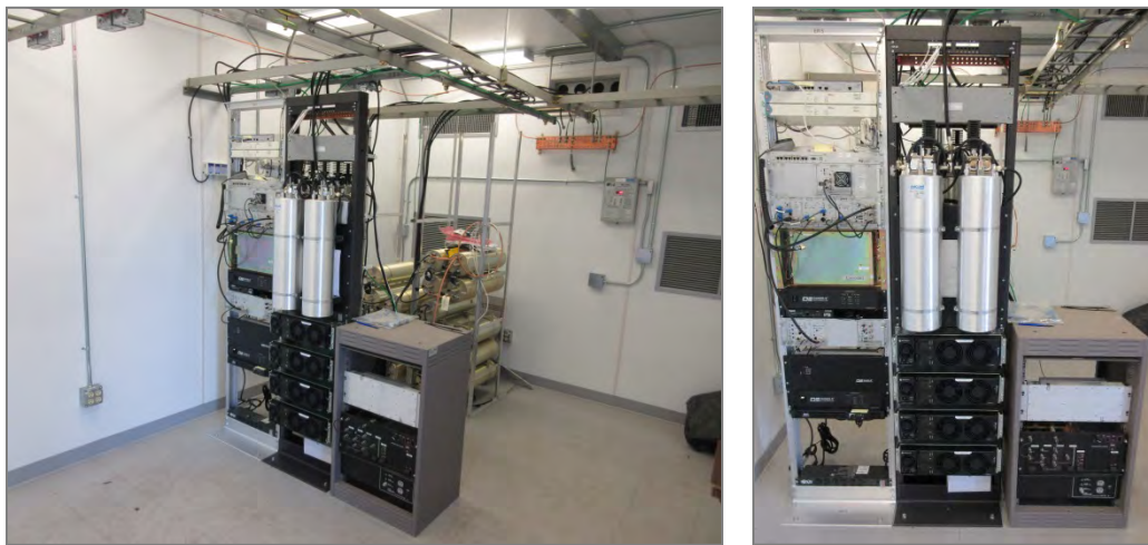
FIGURE 7 Meyers Flats Radio Equipment
