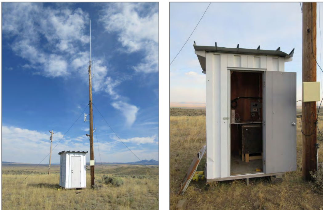
FIGURE 9 Wilsall Mountain Repeater Shelter
