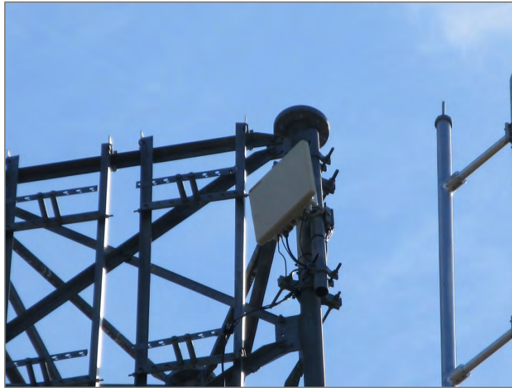
FIGURE 8 Meyers Flats to 9-1-1 Center Microwave Radio and Panel Antenna
