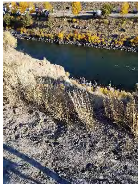
Figure 7 Mile 0.75. Erosion on the fill side above the Yellowstone River.
