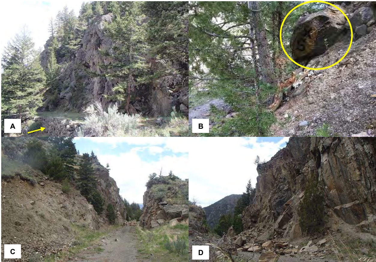
Figure 5 Photographs of rockfall hazards in the Yankee Jim Canyon section (Appendices A-1 and A-4). A) Site US16 looking east (towards Gardiner). The site is along the Yankee Jim Toll Road south sub-section and has historic hand laid drystone rockery wall (yellow arrow). The site has numerous adverse oriented joint sets that allow planar, wedge, and toppling failures. B) Site US17 at the western end, looking east. An historic advertisement painted on a boulder is visible (yellow circle). The slope has unconsolidated silty sand and gravel supporting cobble and boulders. C) Through cut along the road, sites US103 (left) and US104 (right) looking northwest and D) looking southeast. Large rockfall was observed coming off of site US103. Numerous adverse oriented joint sets that allow planar, wedge, and toppling failures.
