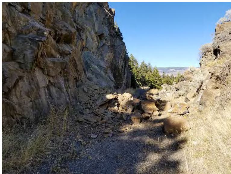
Figure 256 Rockslide at milepost 14.1 looking northwest.
