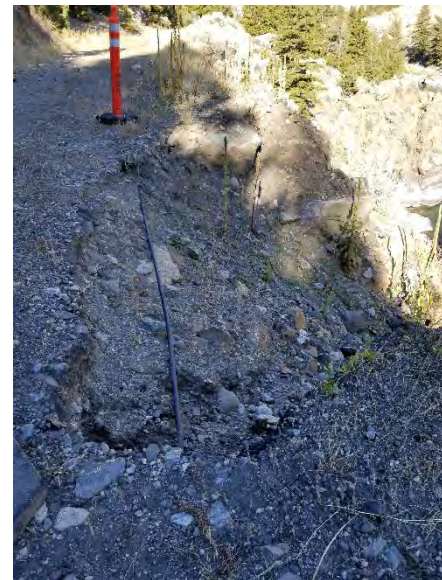
Figure 267 Landslide at milepost 14.2 looking north.
