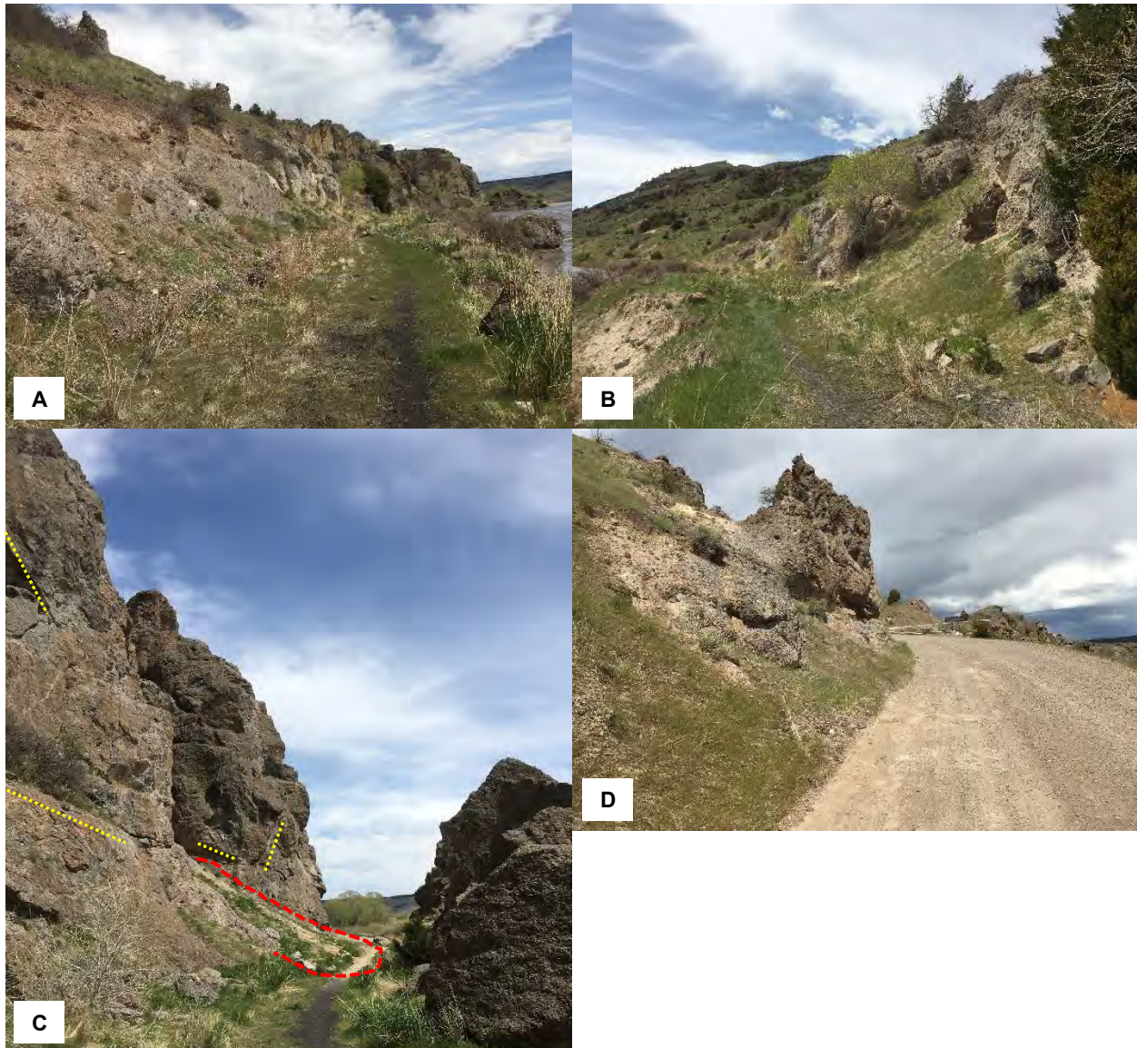
Figure 7 Photographs of rockfall hazards in the Point of Rocks section (Appendices A-1 and A-5). A) Site US19 looking north, with the Yellowstone River on the right. Differential erosion rockfall hazard with a limited ditch catchment along the old rail road grade. B) Site US19 looking south. C) Site US21 looking north. Joint sets are observed in the bedrock (yellow dashed lines) that facilitate planar, wedge, and indeterminate failures off of the 85-foot high bedrock outcrop. A debris flow is observed covering the proposed trail (outlined in dashed red) up to 3 feet deep. The trail curves around the outside edge of the debris fan. Dashed yellow lines highlight joint surfaces, some of which are adverse and consistent with others being indeterminate, or inconsistent. D) Site US110 looking north. Similar Hyalite volcanics as at site US21 (photograph C ).
