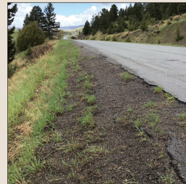
Drainage and Erosion
