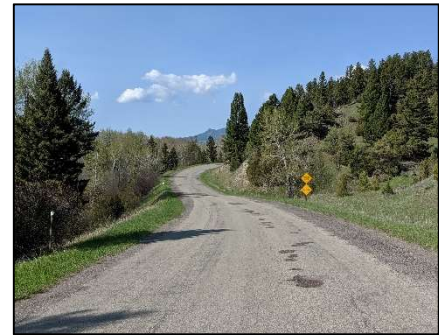
There are safety concerns at MP 6.0 due to steep side slopes, deteriorating roadway edges, and limited sight distance.
