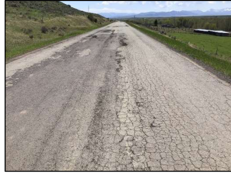
A weak subgrade is characterized by rutting, depressions, or upheaval in pavement. There are several locations along the roadway where the subgrade was noted as being deficient.
