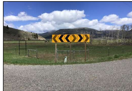
Most of the existing signage at the intersection of Hill Road/Hamilton Road/Shields River Road has fallen over or is missing.
