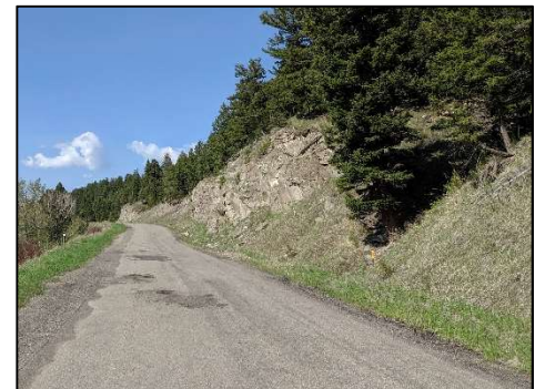
Two landslide areas are documented along the corridor during field review. Slides caused by stream undercutting are also reportedly present in the study area.
