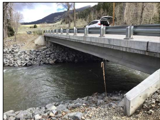
There are four bridges in the study area. All four bridges are in fair or good condition.
