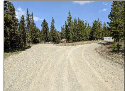
The gravel surfacing is in good condition. General preservation and maintenance should be completed annually to extend the life of the surface.
