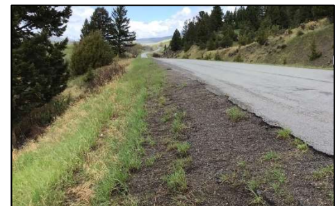
Improper drainage on the roadway can lead to serious erosion issues including deteriorated roadway edges.
